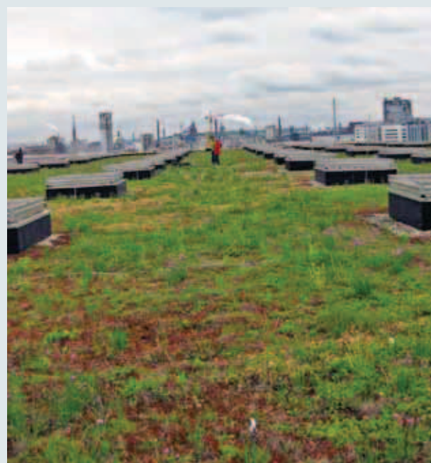
Industry and Ecology in combination: The green roof at the Schachermayer company
